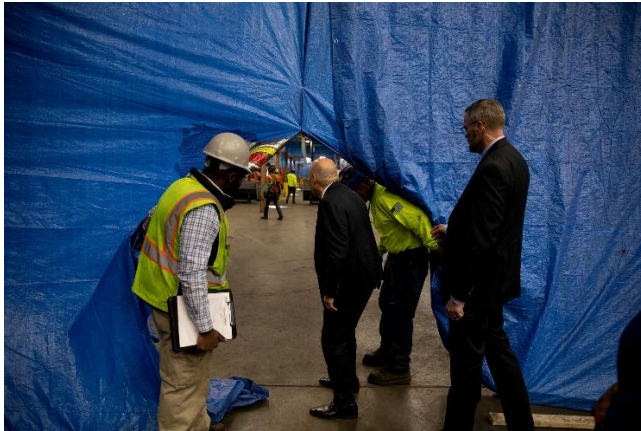
DeJoy surveys construction at the Atlanta processing center Kendrick Brinson for TIME
